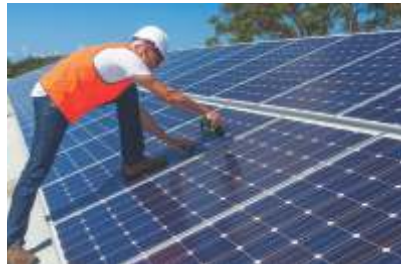
Requirements of the solar industry
